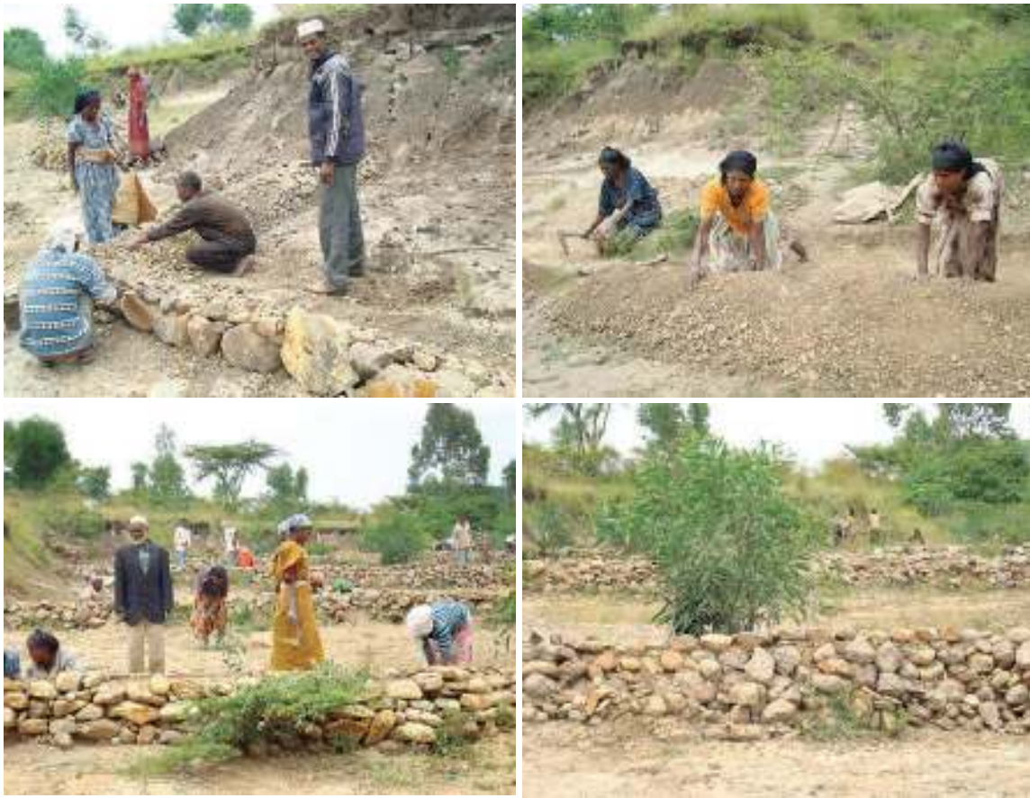
Figure II 18.3 Local people constructing physical soil conservation structures and planting trees and grasses on degraded land at Choroko, Alaba, southern Ethiopia. ©Alaba Agricultural office
